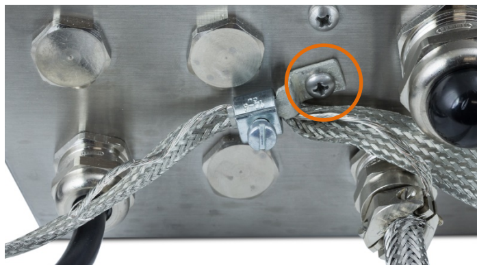
Figure 2-56: Grounding Clamp Mounted to Enclosure
