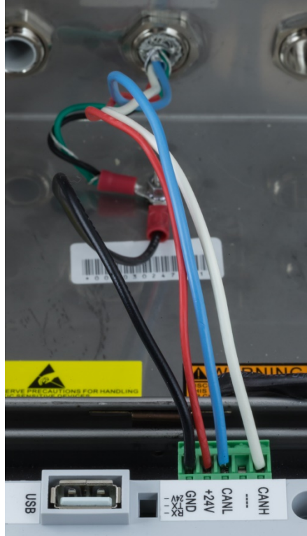
Figure 2-60: POWERCELL Wires Connected in Terminal
