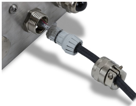
Figure 2-73: Cables Entering Enclosure
